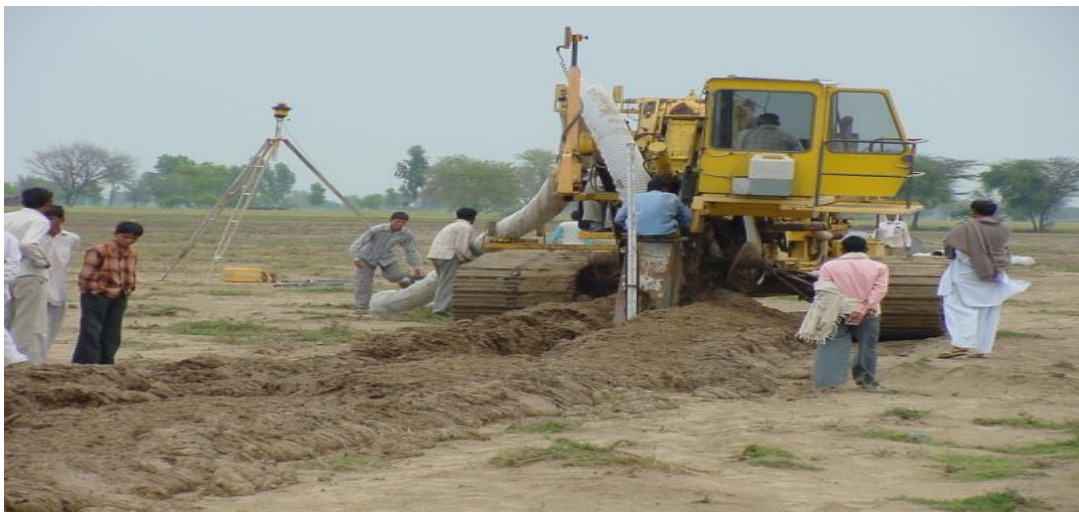
Figure 5. Subsurface drainage system installation in a field of Haryana, India [Source: ICAR-CSSRI reports]
