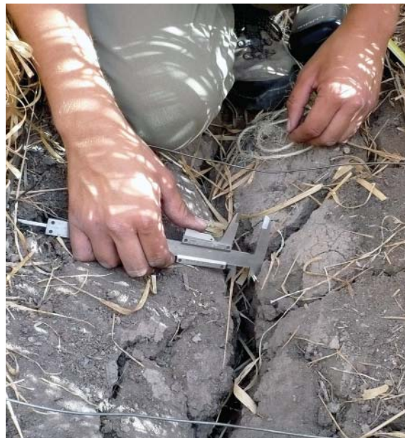
Figure 5. Measurement of crack width.
