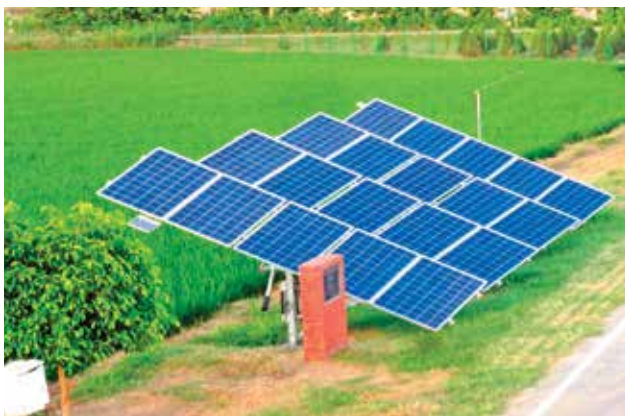
Picture 13. Solar Pumps in the field
